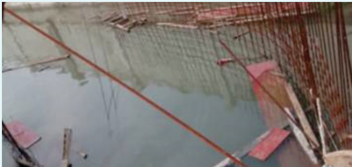
An under construction commercial complex with a loss in excess of Rs. 300 lakhs. Establishing the loss to the satisfaction of the loss assessor when substantial assets had been washed away was an ultimate test of patience for all concerned.
